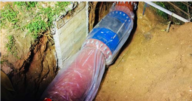
Laid at edge of unstable ground (liquefaction)
