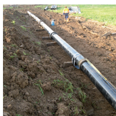
TT PE pipe train ready to be pulled by horizontal directional drilling
